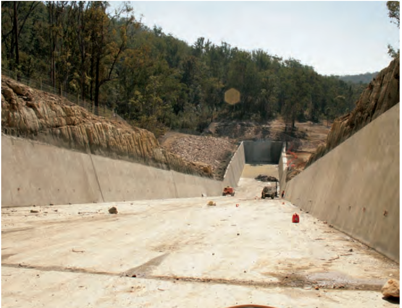
The spillway was excavated in sandstone using drill and blast techniques. The concrete lined section of the spillway was 340m in length and 15m wide at its base.
