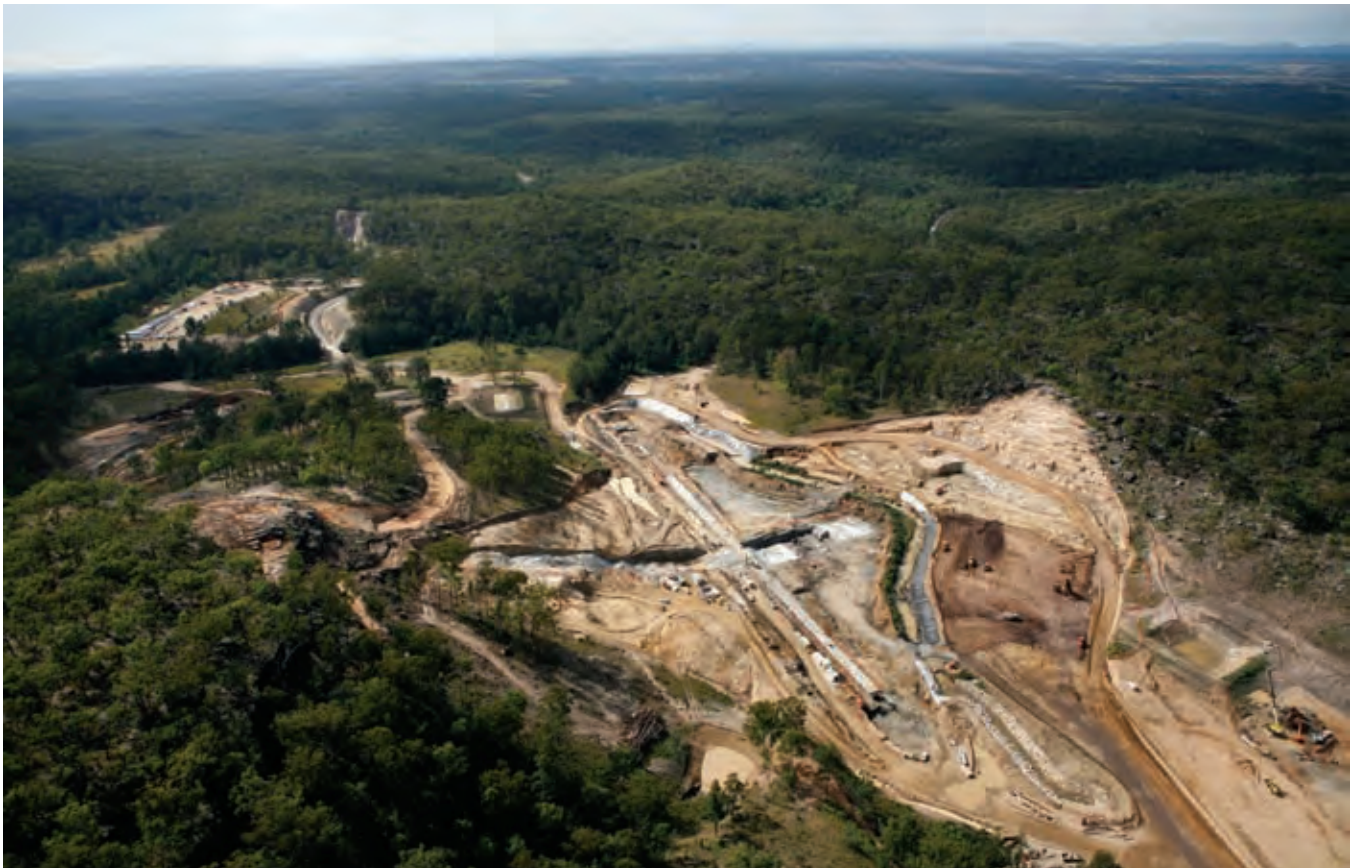
Works progress on the storage facility located within 6100ha of North Coast Water controlled land.
